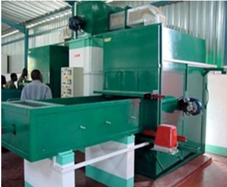
High temperature Incinerator in a hospital
